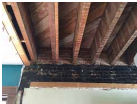
Second floor ceiling joists and the interior of the Jackson Street wall.
