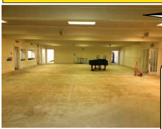
⊕ Thursday, July 7 Carpet removed from Weems Hall in preparation for asbestos abatement.
